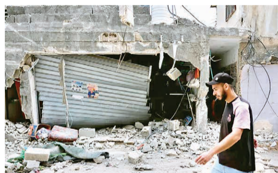
A Palestinian man inspects the damage following an Israeli raid at Nur Shams camp, in Tulkarm, in the Israeli-occupied West Bank.
