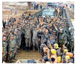
Army completes Bailey Bridge construction in record time, on Thursday. Bridge near Wayanad over Iruvanipzha River connects Chooramala.
