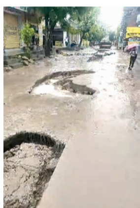
As water subsides, gaping potholes were seen at various places in the city.
