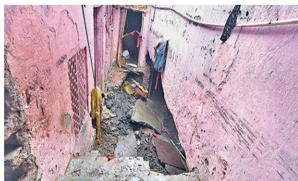
Broken wall and floor that caved in after rainwater entered the basement of a house in VKI area of Jaipur on Thursday. CM Sharma announces financial aid of ₹5 lakh. SUNIL SHARMA
