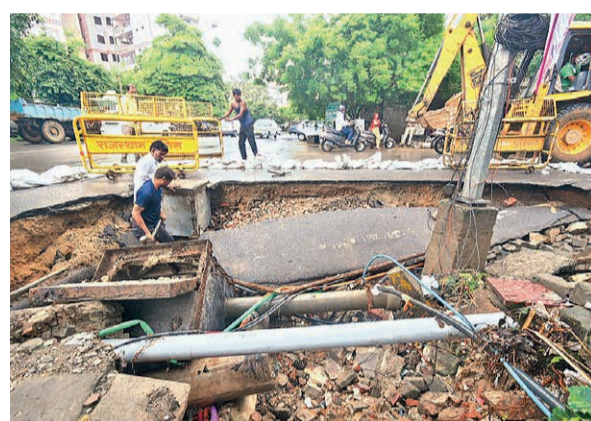
JDA received over 150 complaints of waterlogging, roads caving in and bursting sewer lines in city throughout the day.
