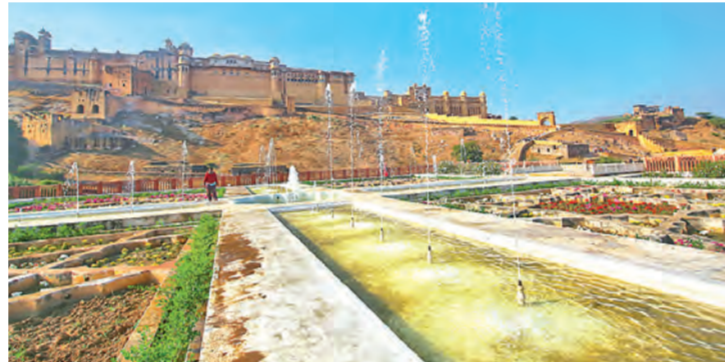
Fountains are being checked and repaired at the Kesar Kyari near Amber Fort in Jaipur on Sunday. SUNIL SHARMA
