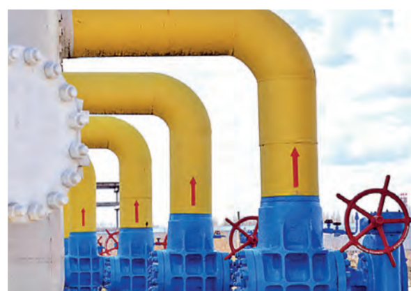
A gas worker walks between pipes in a compressor & distribution station of the Urengoy-Pomary-Uzhgorod gas pipeline. FILE
