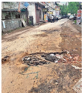
The damaged roads in Ram Nagar area.
