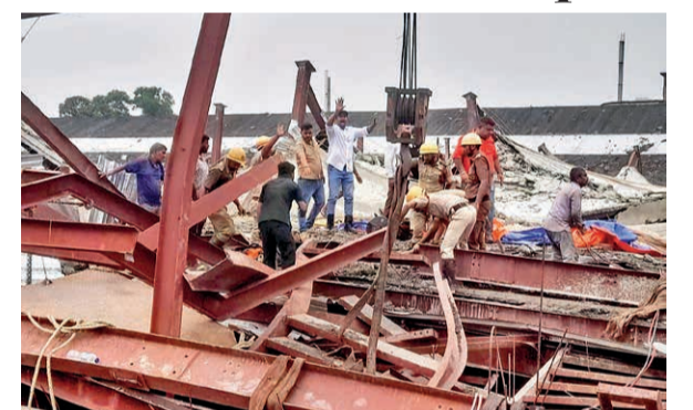
Search and rescue operation underway at the site where an under-construction godown shed collapsed in Taratala, in Kolkata, West Bengal, on Wednesday. PTI
