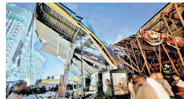
A hoarding collapses in Mumbai's Ghatkopar area on Monday.
