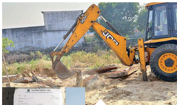
A bulldozer demolishes illegal colony Kanota Anand near Kanota on Agra Highway in Jaipur.
