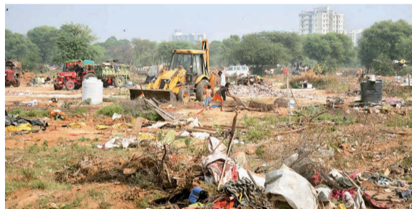
A bulldozer demolishes illegal constructions in between Akshay Patra and NRI Circles in Jagatpura area in Jaipur on Tuesday.
