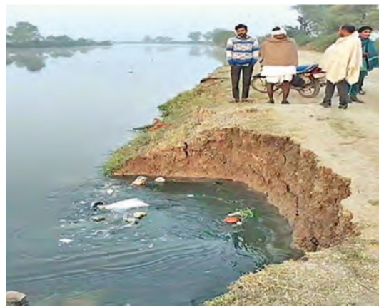
Water leakage has been reported from the escape section of the Chambal's right main canal.
