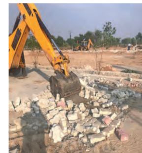
walls, being built without JDA approval. The action follows similar efforts in Zone-11, where two illegal colonies were also dismantled. In a separate action, JDA also freed 7 bighas of govt land in Bagru from illegal encroachments, including tin sheds and wooden structures.
