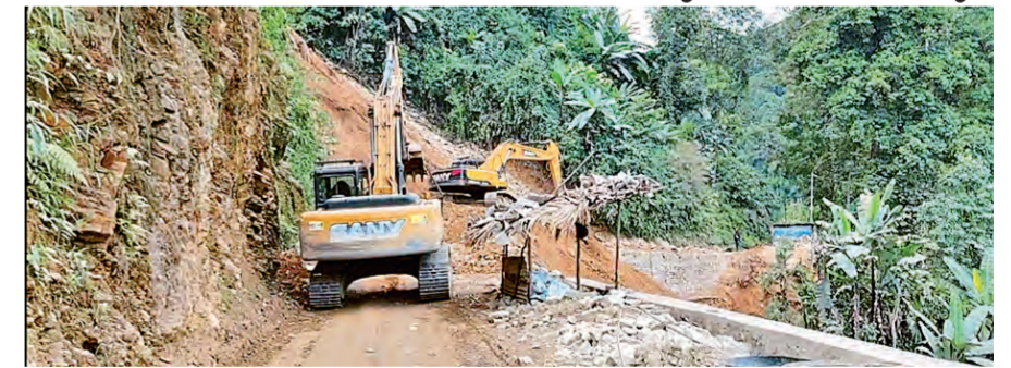
As the BRO continues to enhance infrastructure in Arunachal Pradesh, these efforts are not only crucial for national defence but are also playing a pivotal role in uplifting the local economy and improving the standard of living of residents in this challenging terrain.
