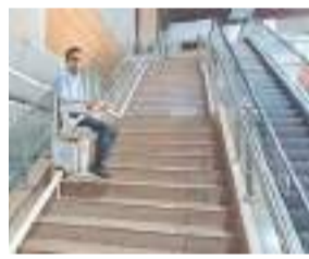
Automated Stairlift at T2.
